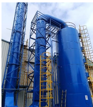
PTIC Lead Fume Purify System
