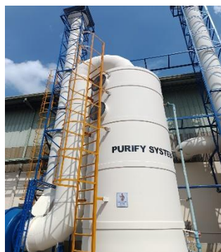
PTIC Acid Fume Purification System
