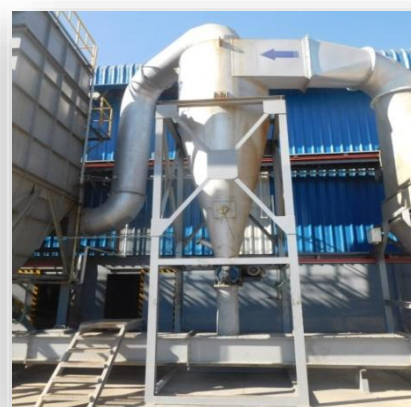
YMI Exhaust (dust & gas) Settling & Cooling Chamber
