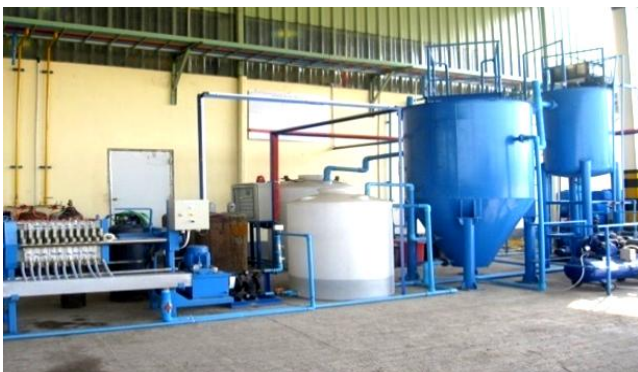
Centralized Waste Water Treatment
