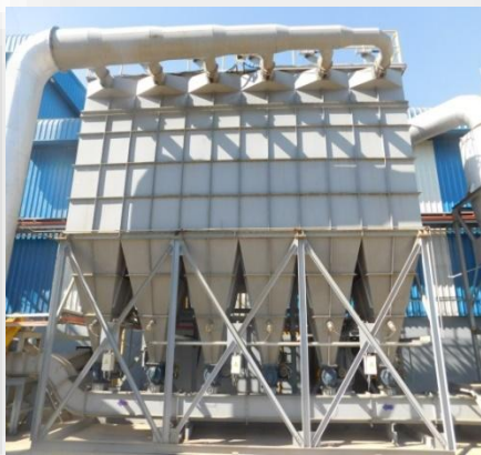
YMI Bag House to filter lead dust from Rotary Furnaces
