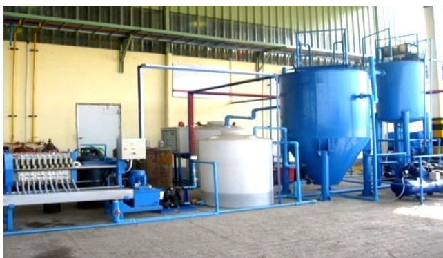
Centralized Waste Water Treatment
