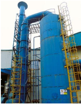
PTIC Lead Fume Purify System
