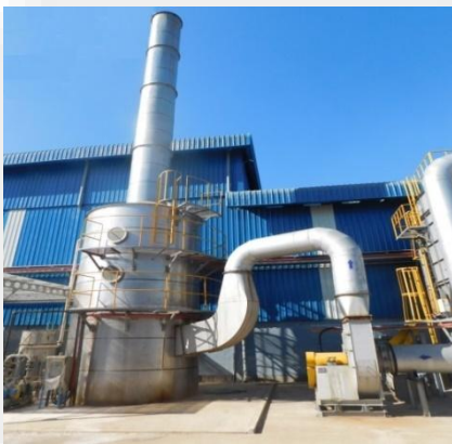
YMI Blower and Wet Scrubber for gas Neutralization
