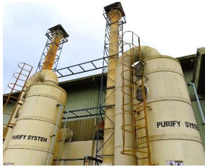
PTIC Acid Fume Purification System
