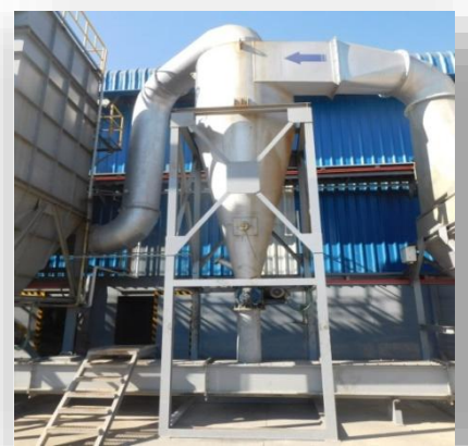
YMI Exhaust (dust & gas) Settling & Cooling Chamber
