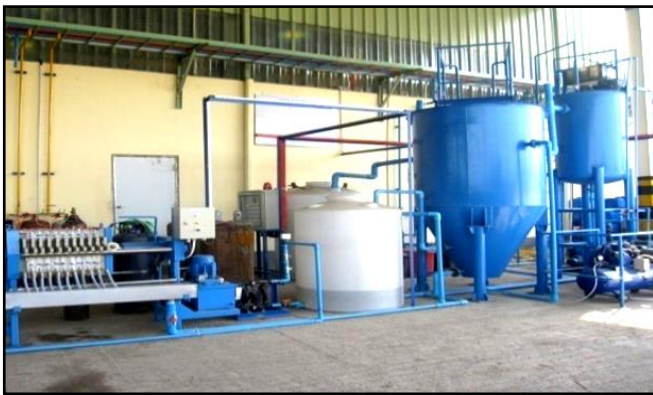
Centralized Waste Water Treatment
