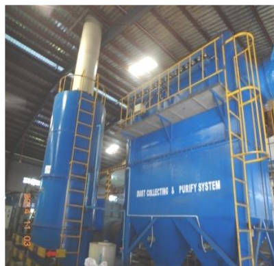
Dust Collector Machine
