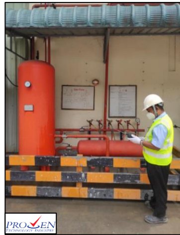
Gas Leakage Monitoring
