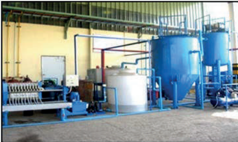
Centralized Waste Water Treatment
