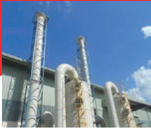
Lead Fume Purify System
