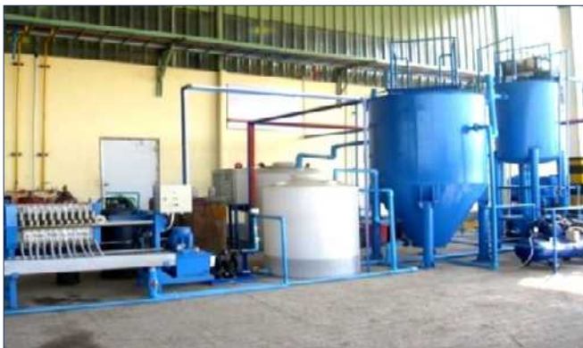
Waste Water Treatment Plant
