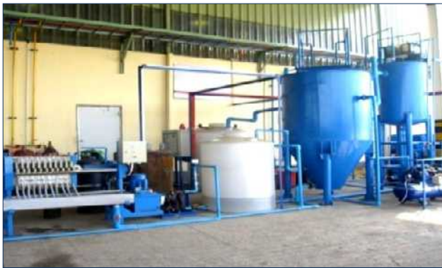
Waste Water Treatment Plant
